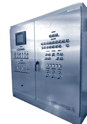
■ Control panel for the plant.
