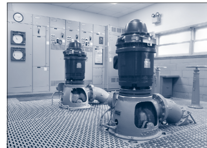
Pump Station at Lourae Drive
