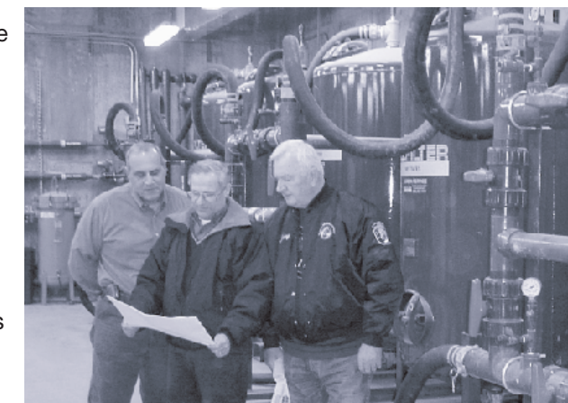
Water filter systems located at the Liberty site.
